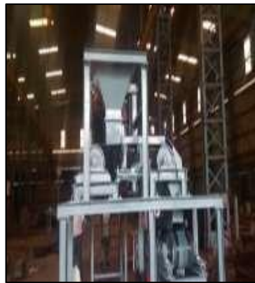
Conveyor with flowability setup
