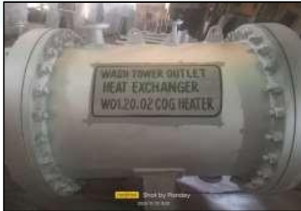
HEAT EXCHANGER- COG HEATER
