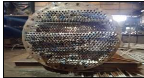
IN PROCESS SS TUBE WELDED HEAT EXCHANGER
