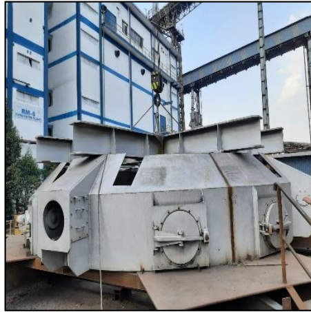
LCP On Site Assembly Condition After Supply
