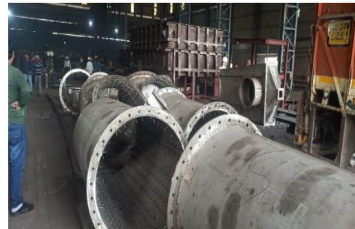
SS Material - Car Modified De-dusting System - Unique Engineers
