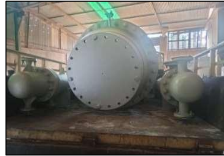
HEAT EXCHANGER LOGISTICS
